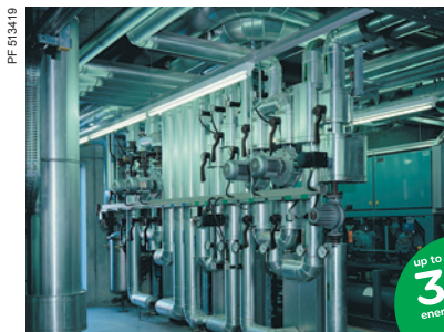
ATV12 controlling a pumping station
